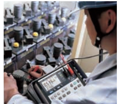
3551 Checking the battery in an Uninterruptible Power Supply (UPS) without shutting down
